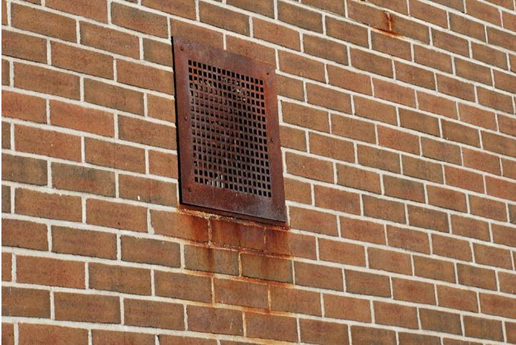
Exterior walls at the Savage Center show the results of no weeping system or cavity wall construction
