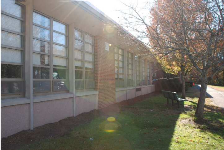
A portion of the infill pre-cast panels along the exterior envelope are designed with an intake grille for mechanical ventilation
