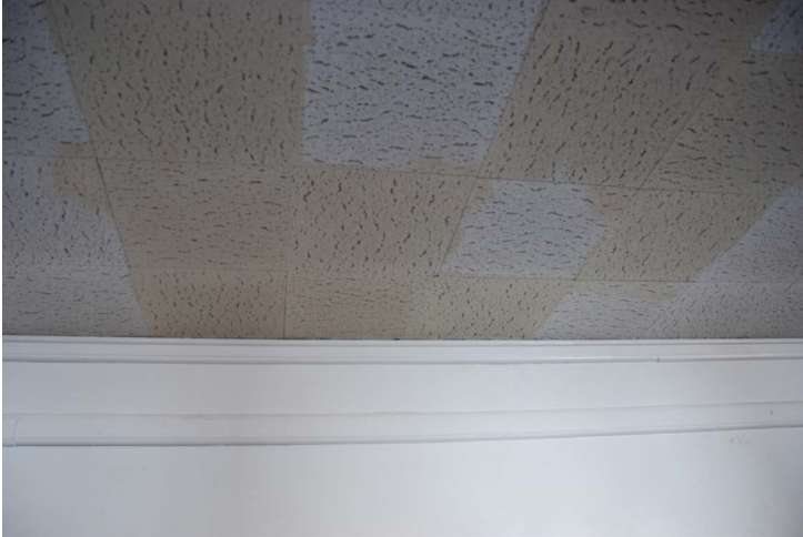
The main floor corridors are finished with Asbestos Ceiling Tile, a hazardous material, that show signs of water damage
