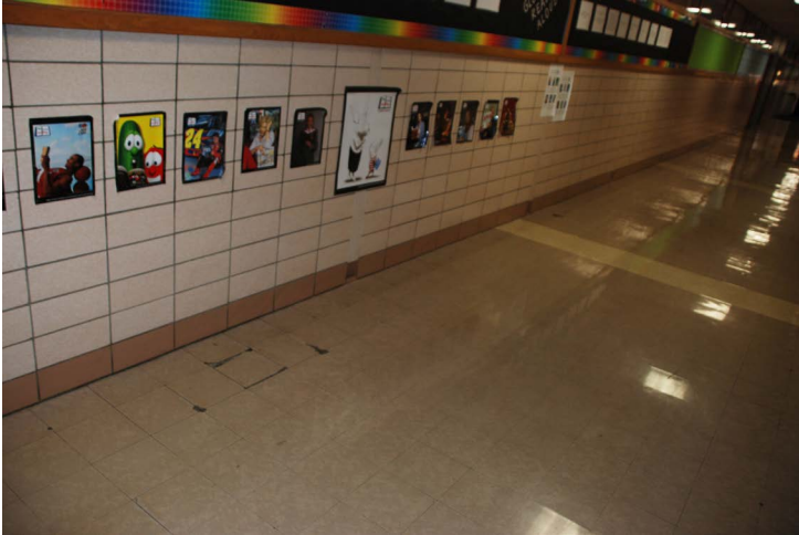
The Vinyl Asbestos Tile (VAT) throughout the corridors is a hazardous material that will cause harm upon degradation
