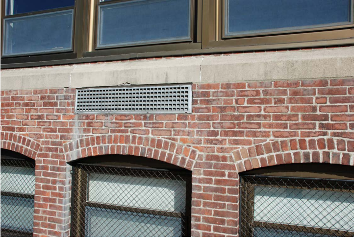
The appearance of a white-colored deposit over the surface of the exterior brick may be efflorescence
