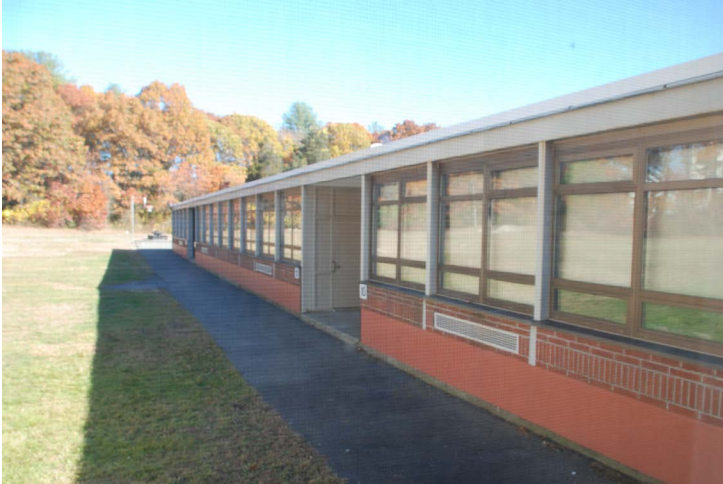
Due to the change in grade between the three winds, exposed foundations walls are obvious
