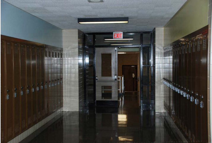
The corridors are a mismatch of finishes between brick, plaster, and glassed tile; all lined with obsolete lockers
